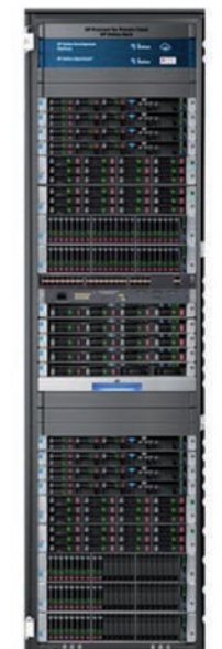
Fig. 6 - HP Helion Rack
